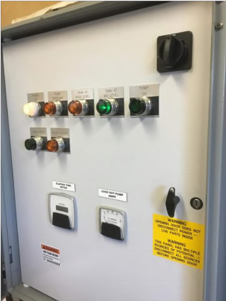
1 EXISTING TANK NO.4 PUMP AND VALVE CONTROL PANEL NOT TO SCALE
